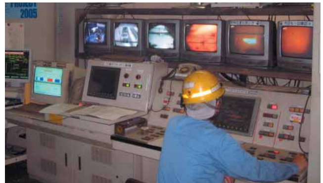
Central Control Room
