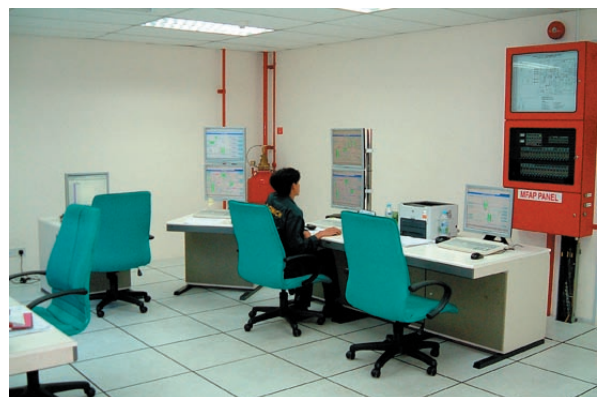
Central control room
