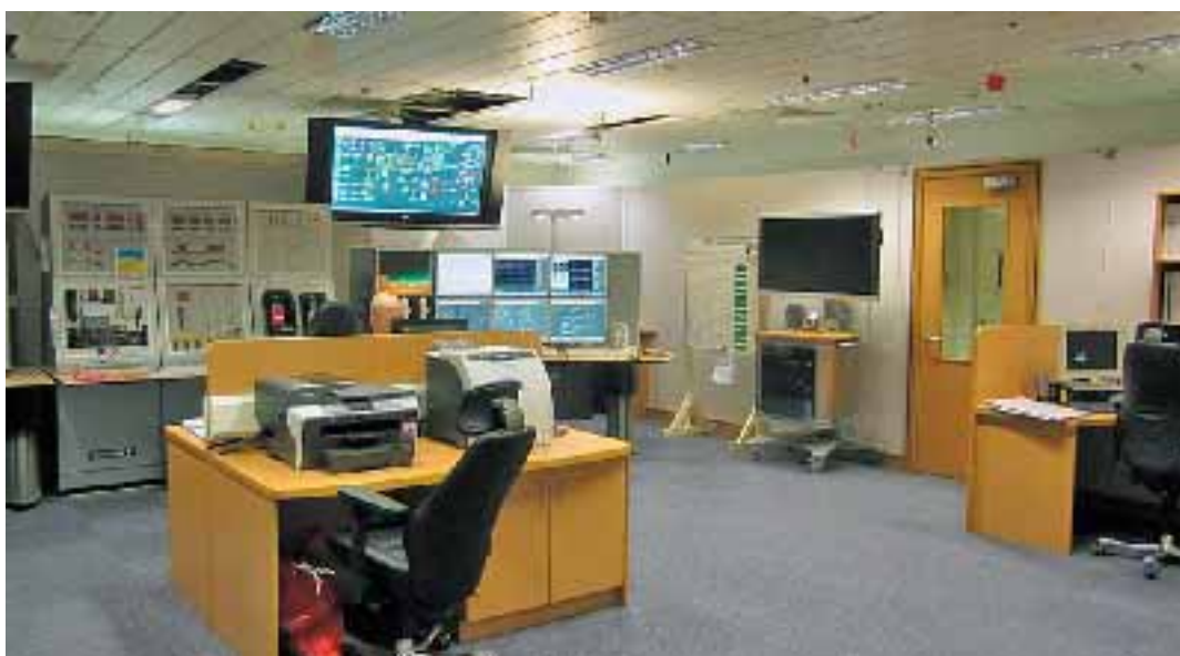
Bruce control room
