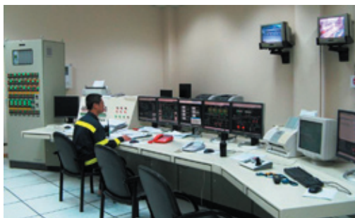
Central control room
