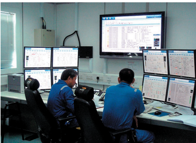
Central control room
