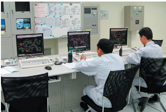
During plant commissioning
