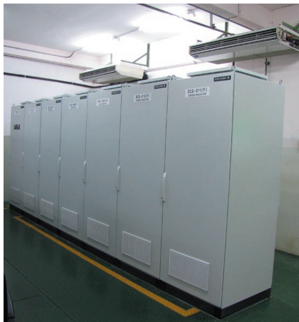
Rack room: clean and neat
