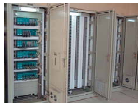
FCN Controller & Panel
