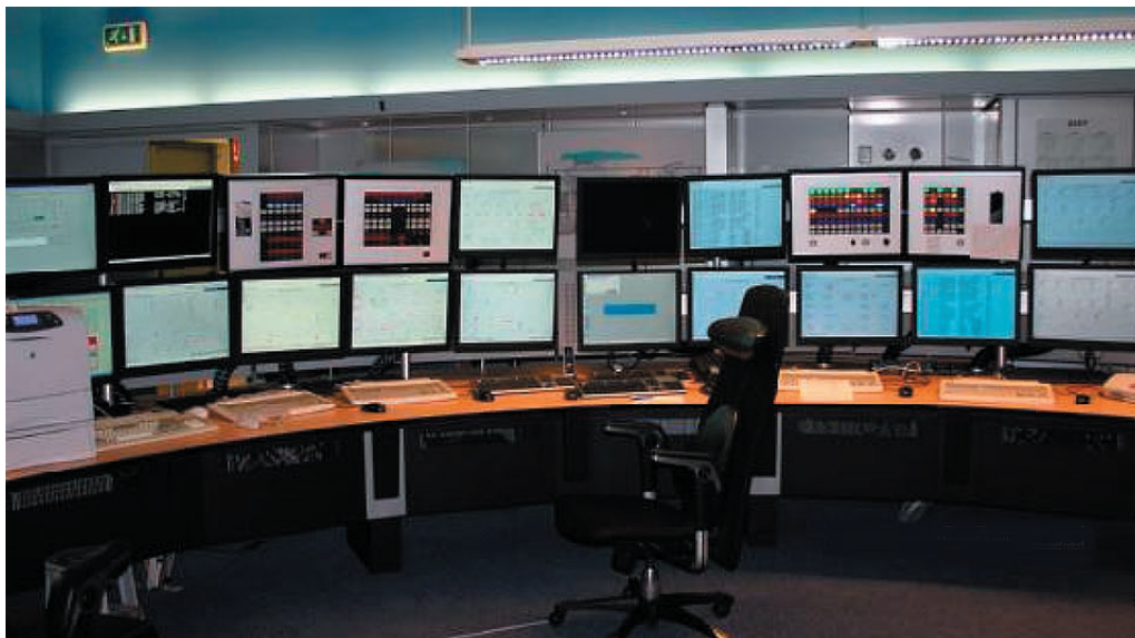
Central control room at Den Helder
