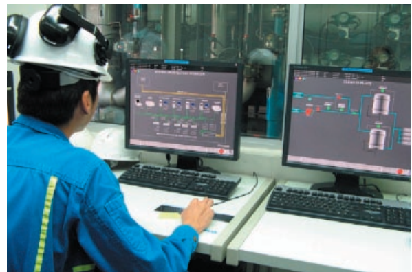
Main control room for field operations
