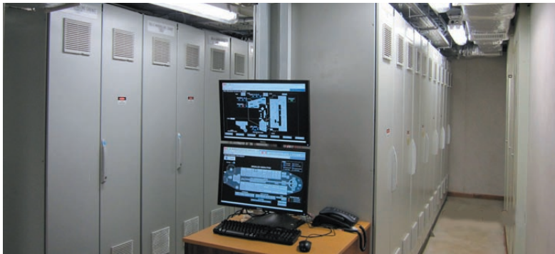
Instrument technical room
