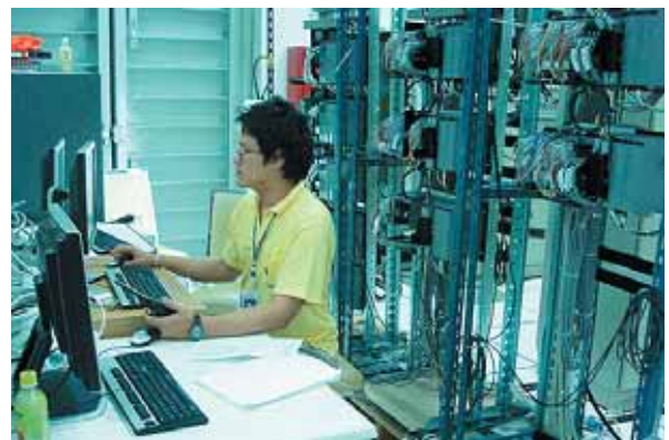
Field control station SAT in rack room
