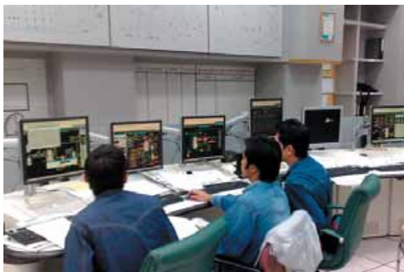
Human machine interface SAT in main control room
