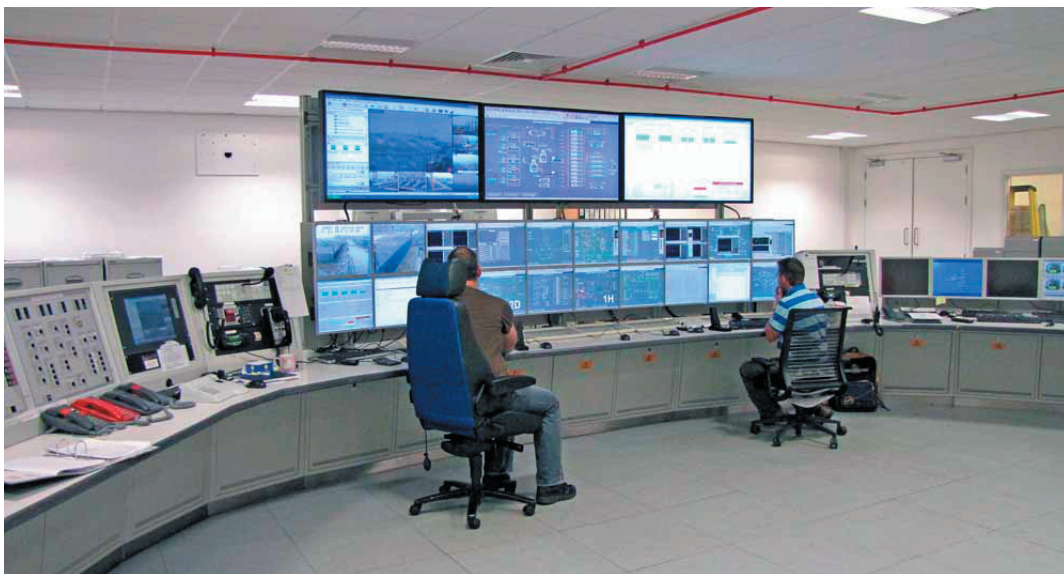
Central control room
