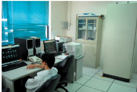
Central control room
