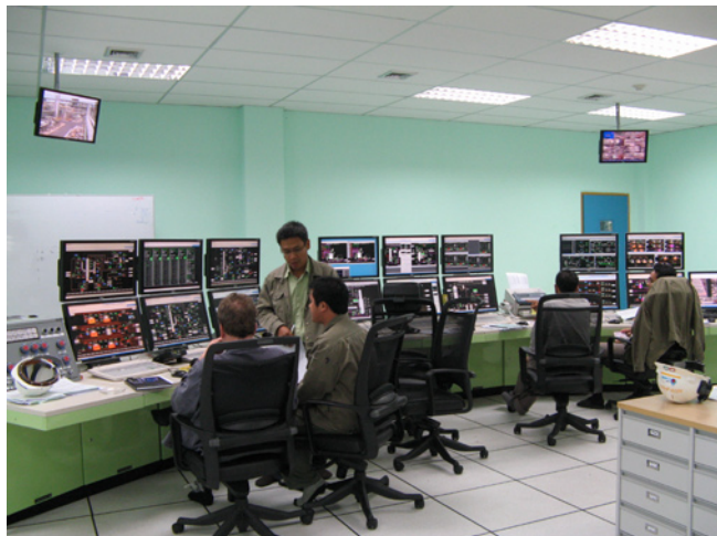
Main control room
