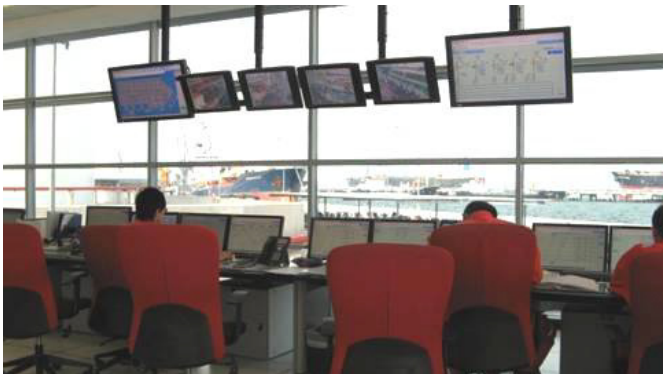
Central Control Room
