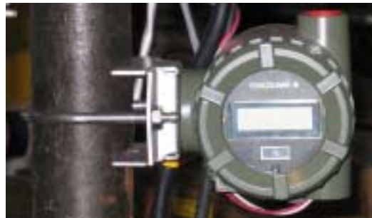
MLD – Digital Loop Indicator
